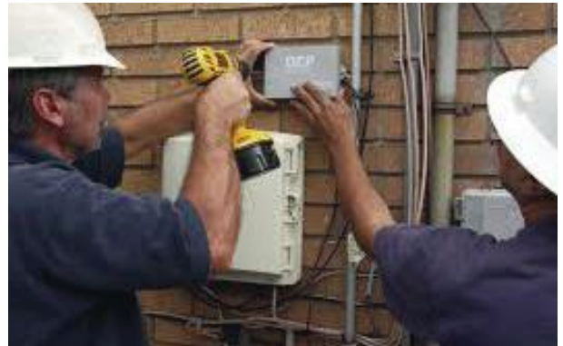
3. Data collector units forward information directly to New York City's Department of Environmental Protection through Ethernet connections to the city's NYCWiN wireless system. (Courtesy of SLive.com)
